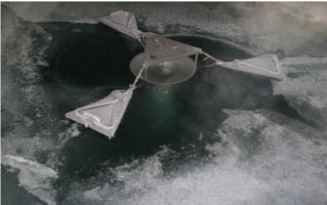
Figure 4. Holes can be broken through ice up to about 0.2 m thick to install a SolarBee mixer.
